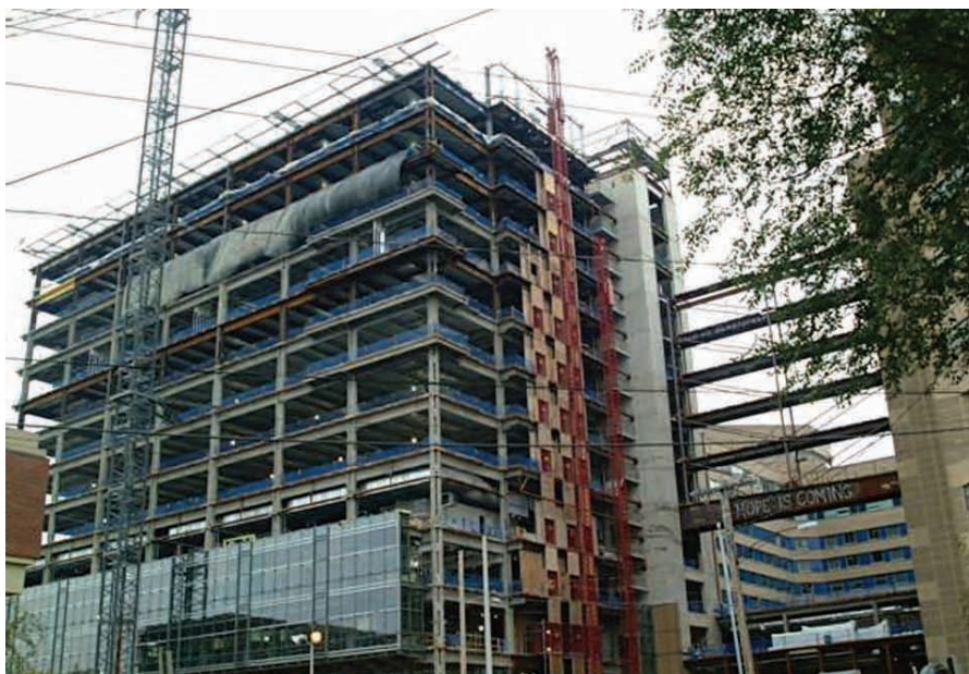
A photo of the The Smilow Cancer Hospital taken on September 9, 2008. The opening date of the Hospital is scheduled for October 26, 2009. We hope that many of you can join us for the celebrations.
